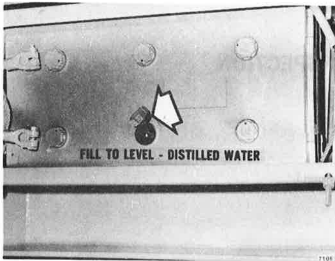
Figure 82 ELECTRICAL STORAGE BATTERY
